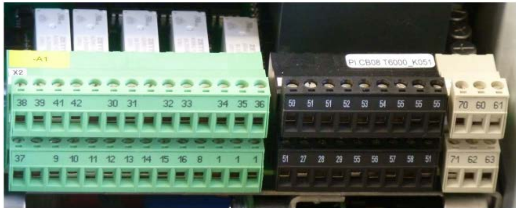
Figure 8-13 Control cable terminals
