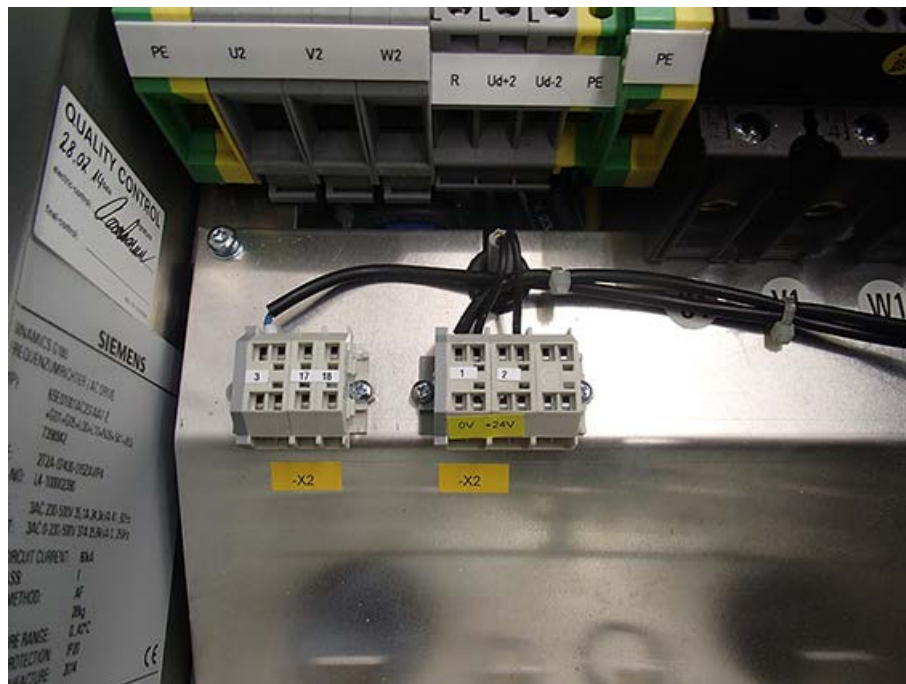
Figure 6-5 Connection for external control voltage
